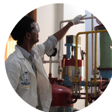
Bio-diesel plant 50 L Capacity
